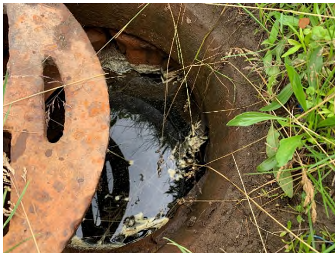
CB – 2 (Catch Basin)
