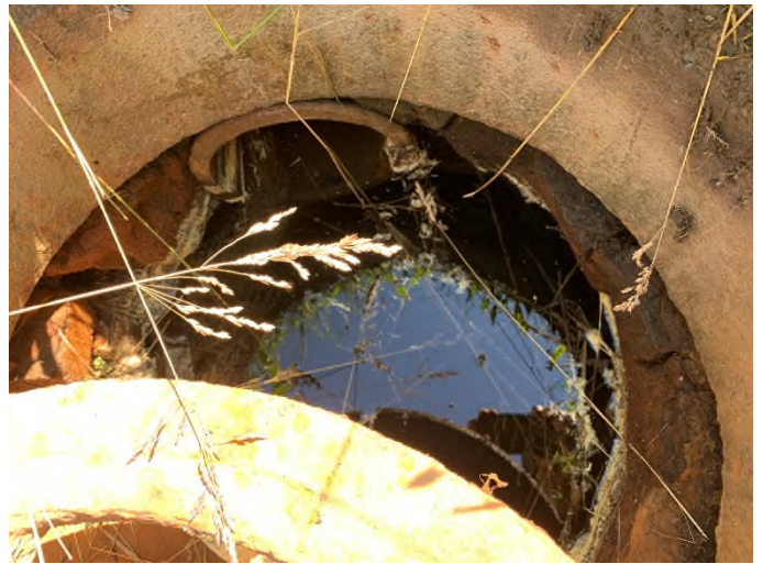
CB - 2 (Catch Basin)
