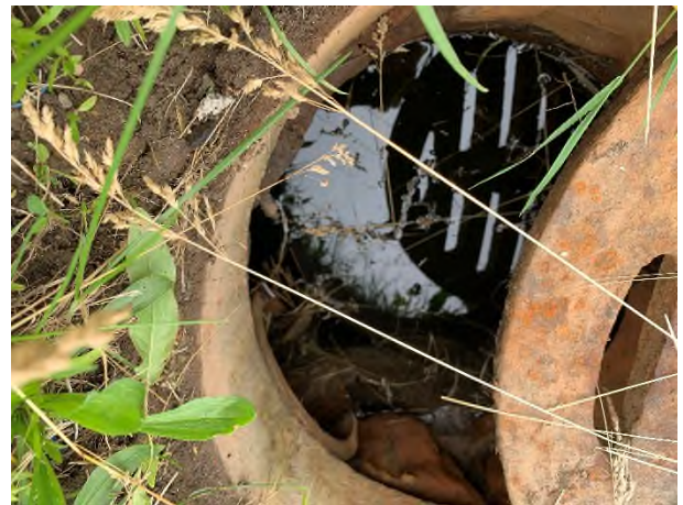
CB – 2 (Catch Basin)
