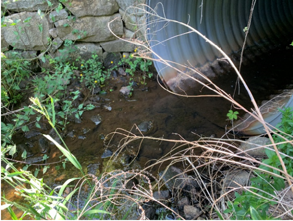
Reservoir Brook – 1 (Brook)
