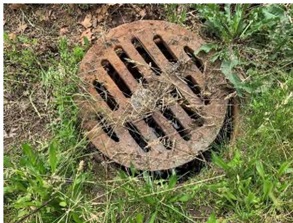
CB – 2 (Catch Basin)
