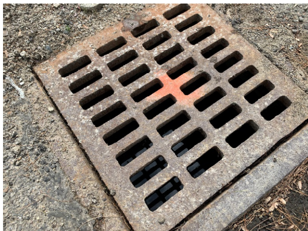
CB – 1 (Catch Basin)
