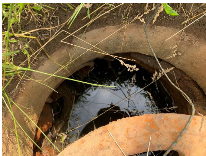
CB – 2 (Catch Basin)
