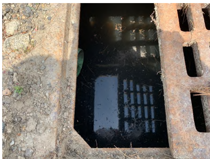
CB – 1 (Catch Basin)
