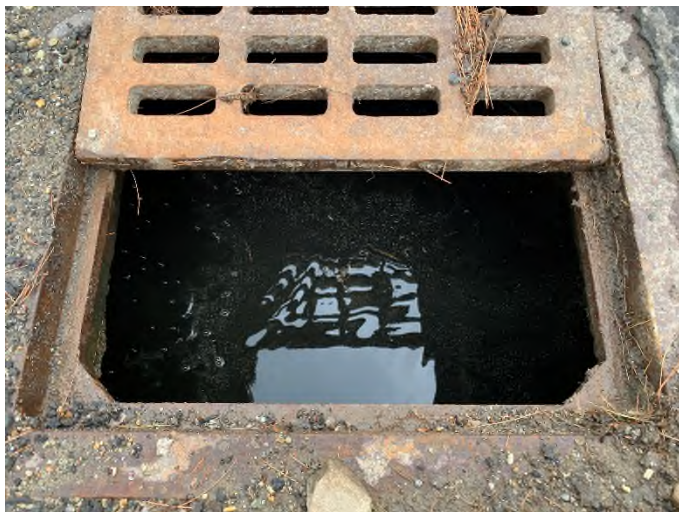
CB – 1 (Catch Basin)
