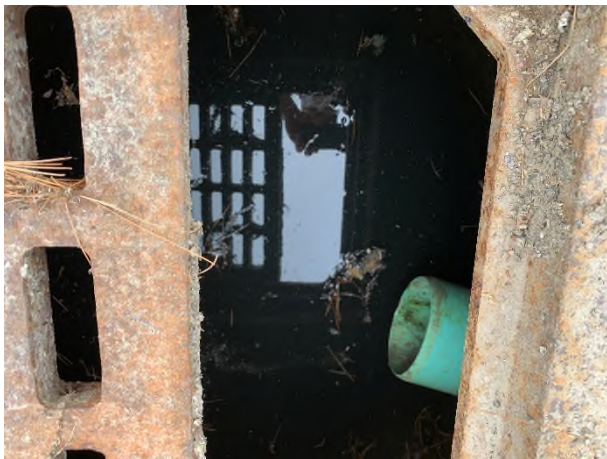
CB – 1 (Catch Basin)
