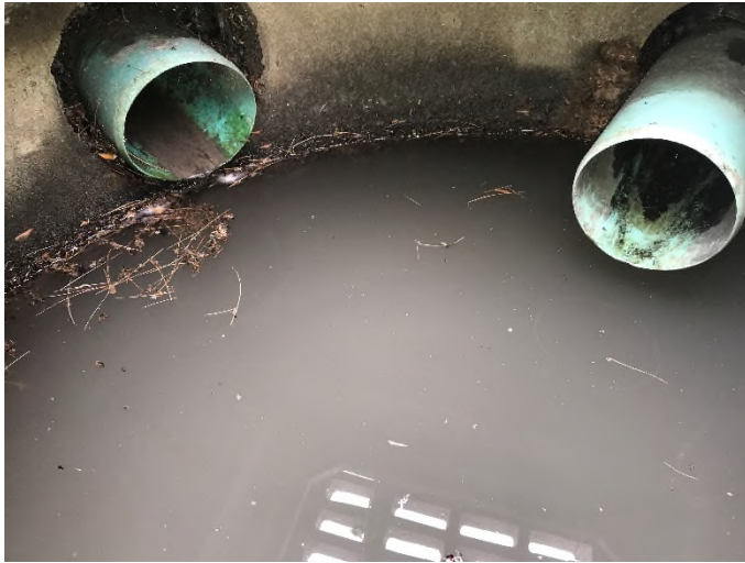
CB – 1 (Catch Basin)
