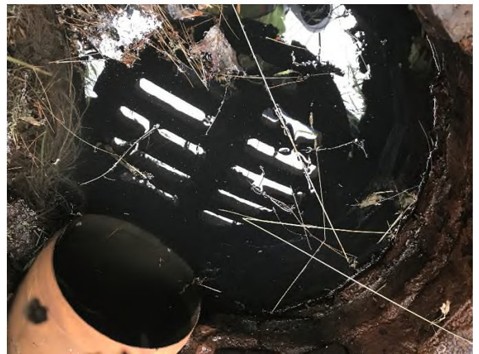
CB – 2 (Catch Basin)
