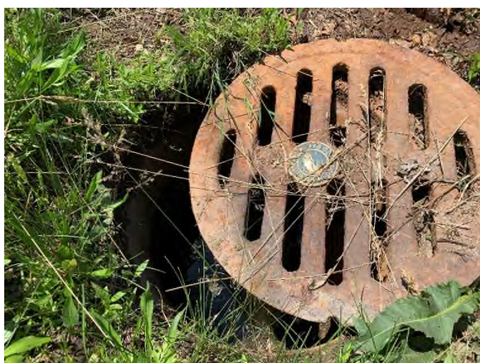
CB – 2 (Catch Basin)
