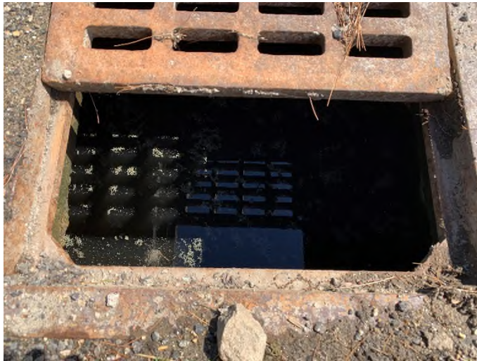
CB - 1 (Catch Basin)
